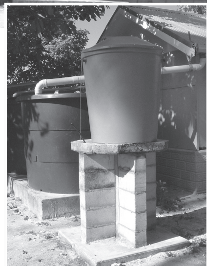
Support water tanks
