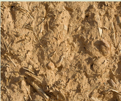
A close up photograph of a mud used to make the wall.
