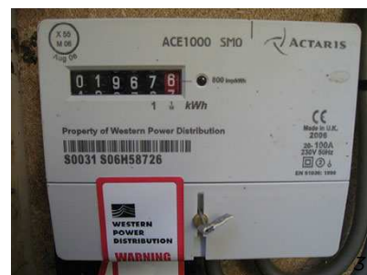
An electricity meter. Can you see the number recording the electricity usage in kilowatt hours (kWh)?
