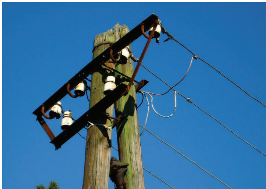
In this photo, the wooden poles and white ceramic caps are electrical insulators.
